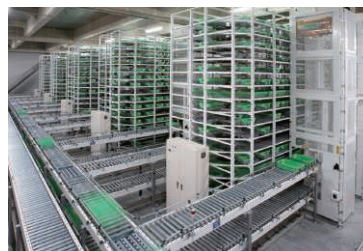
Rotary racks and conveyors
